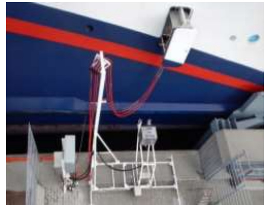
Quay side interface while connected to ship
